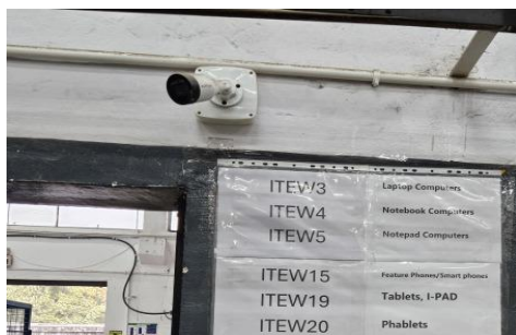
CCTV camera and list of e-waste items
