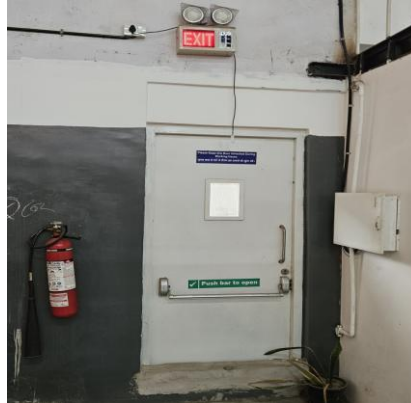
Emergency exit with fire extinguisher
